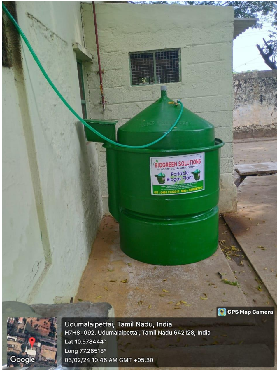
BIOGAS PLANT VIEW 1
